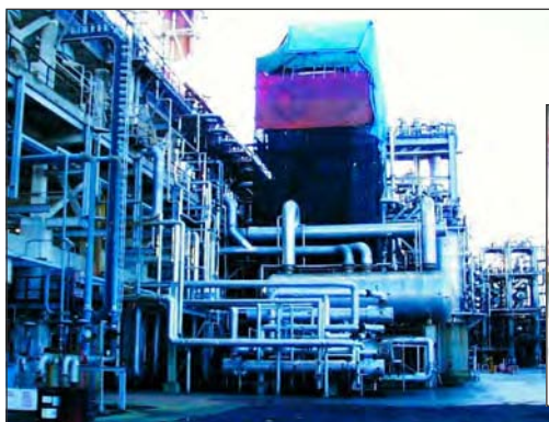
INSULATED INSTALLATION APPEARS SOUND
